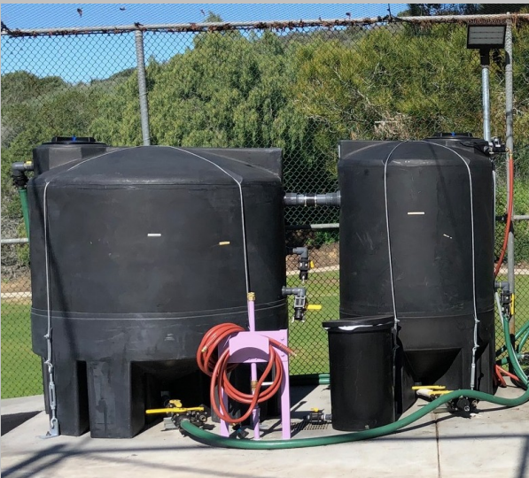
CLARIFIER & WATER STORAGE
